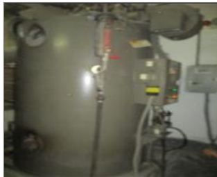
Photo of the inside of the main production hall Boiler.JPG
