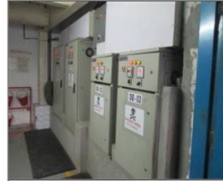
Photo of the inside of the main production hall LT panel.JPG
