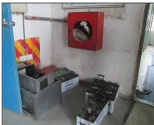
Photo of non-conformity Batteries kept closed to hose pipe.JPG
